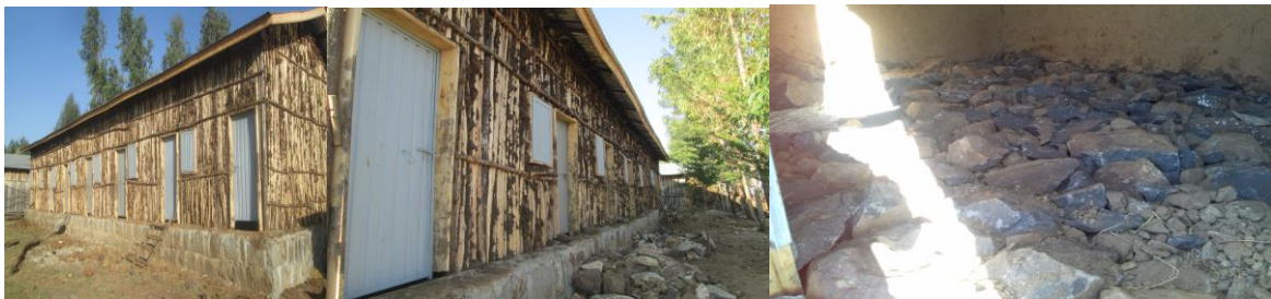
The front and rear view of Teachers Residence and partial view of a room with filled stone
