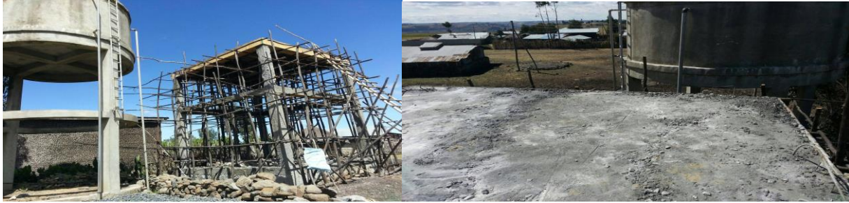
The water tanker stand and the concrete slab of the seat for the tanker beside the old water tanker
