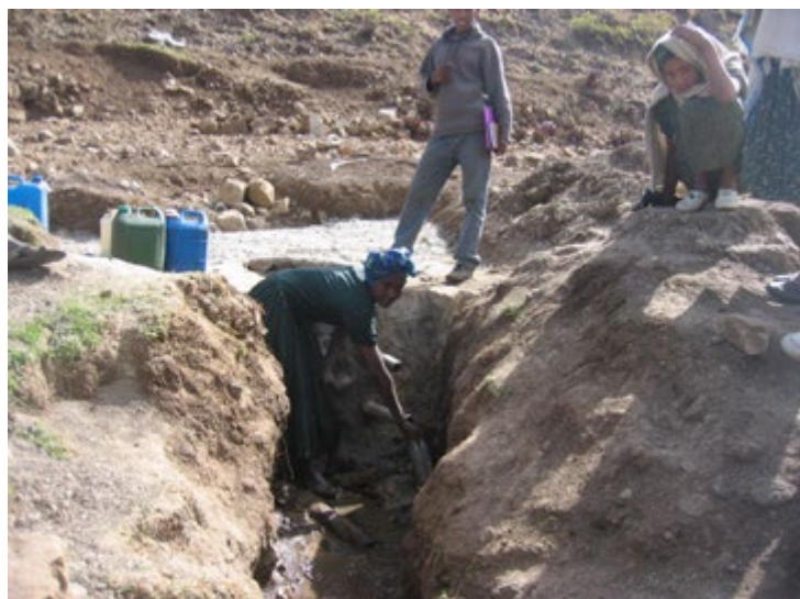
Local woman using water source that is being developed at Metkoria
