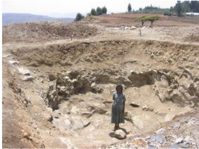
Water collection pit
